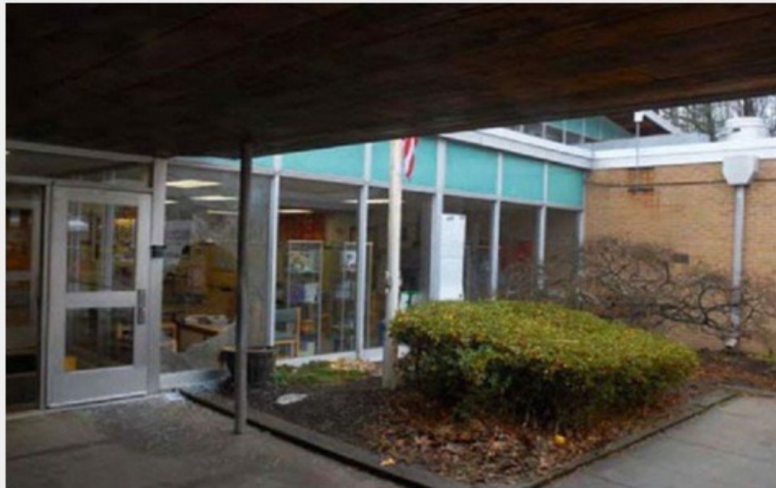
Outside view of shattered glass window
