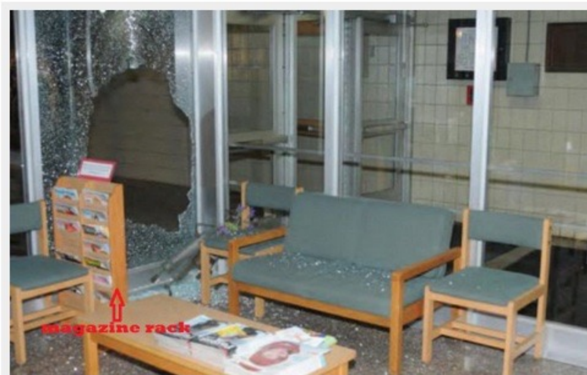
Inside view of shattered glass window and wooden magazine rack on left
